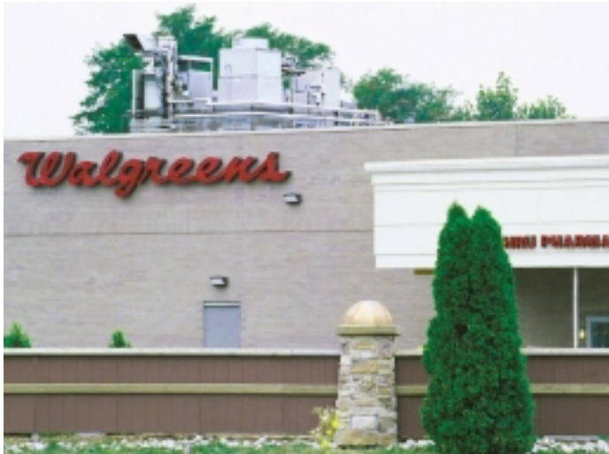
Walgreens recently installed a natural gas microturbine.
